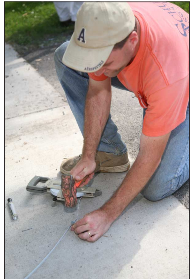
Curt hammers a special masonry nail with a folded yellow tab underneath into the sidewalk along the street, to establish the location where the corner of the lot was found. (He was directed to the proper location via directions received from readings made by Rich.) The nail has an indentation in the center, which provides an easy location to place and hold the point of the prism pole.
