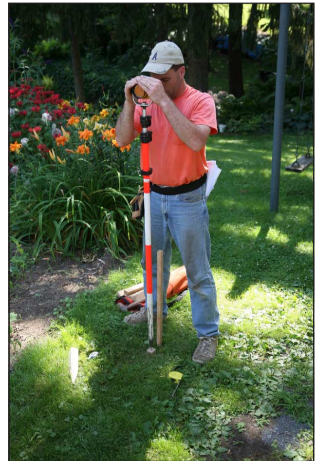
Curt establishes the rear corner of the garage. Since this is the side of the garage closest to the lot line it is important to ascertain that the construction conforms to the zoning requirements.
