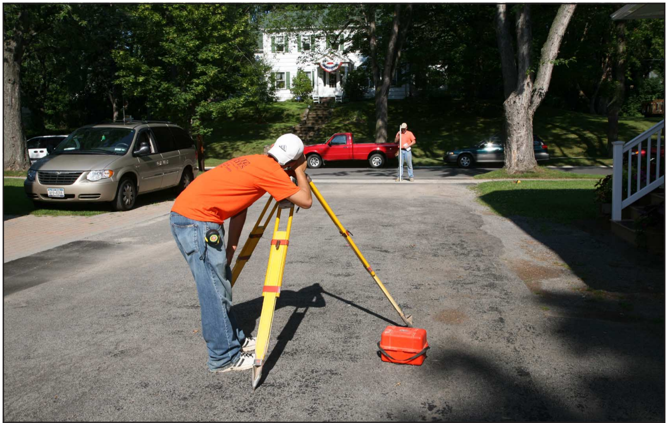
Rich switches to level mode on the Total Station to determine the height of the garage sill. The aim was to set the floor of the garage at an elevation which promoted positive drainage.
